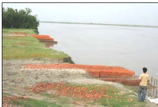
A Vulnerable stretch on the western embankment
