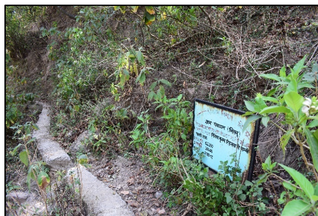
Damaged kuhls, Maniyana village, Dharamshala (Gaj II)
