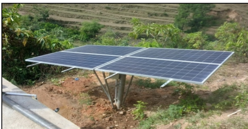
Solar lift scheme in Village Matela
